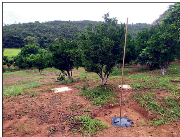
Figure 7. Septic tank installation set (tank, drying bed and sinkhole)
